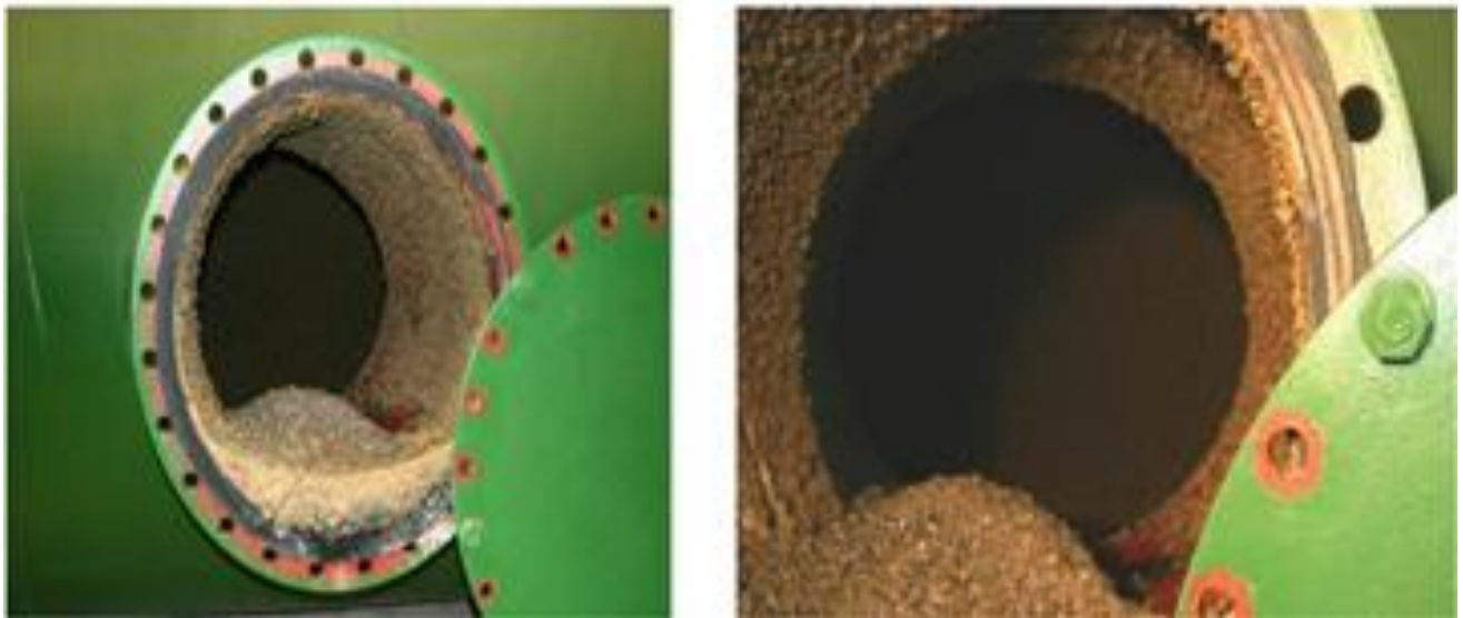
Figure 15. Zebra Mussel accumulation in Şanlıurfa City raw drinking water supply pipe.(21).
