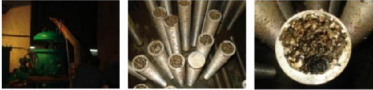
ATATÜRK Dam HEPP Cooling system
