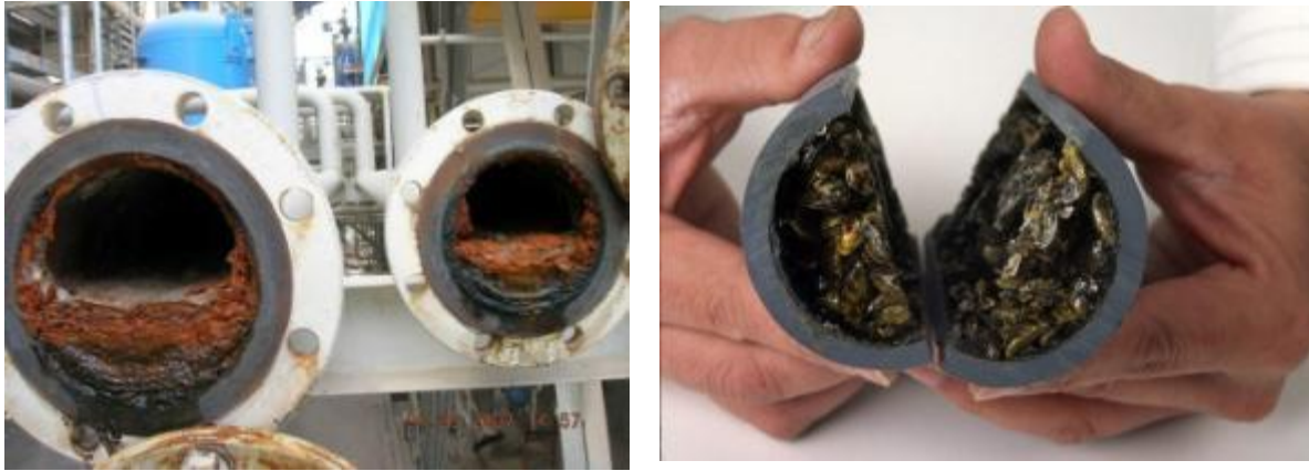
Figure 16. Zebra Mussel accumulation in the pipes.
