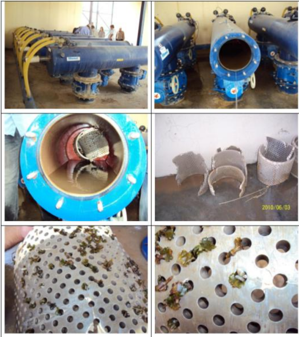
Figure 13 .Urfa Bozova Irrigation Pump Station's Filters in 2010 (21)
